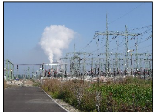
Power and distribution
